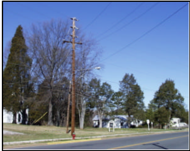
Figure 7: Typical utility pole with overhead lines and street light.
