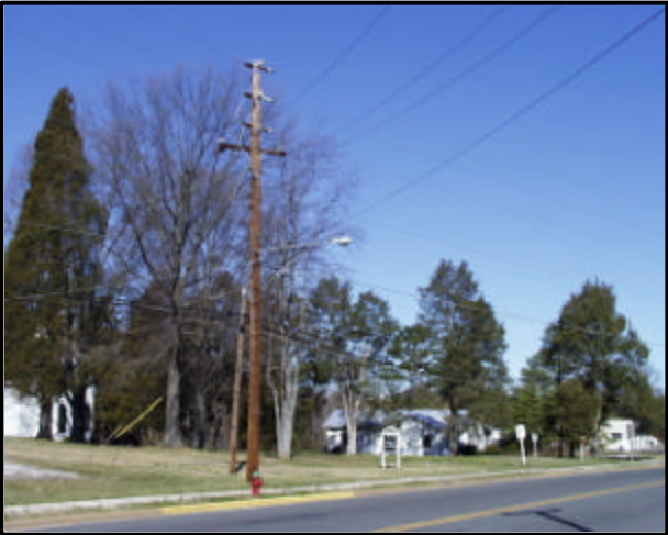
Figure 7: Typical utility pole with overhead lines and street light.
